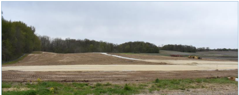
Development in progress of the IMPA solar field in Columbia City, May
