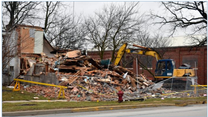
Demolition of an unsafe building on South Main Street in March, Columbia City
