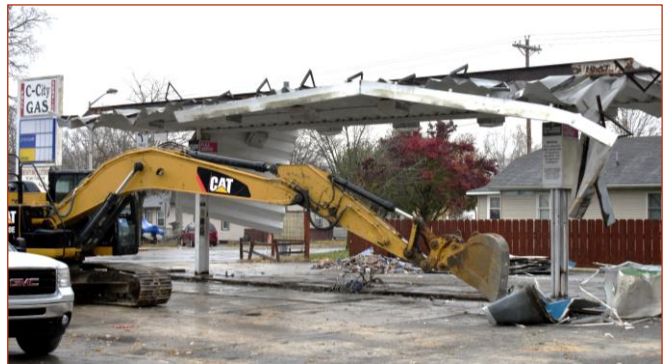
Demolition of the C-City Gas in Columbia City in November. This had been the last full-service station in the County, but closed due to a failing structure.
